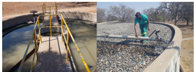
Figure 1: Underperforming wastewater treatment plants in the Phalaborwa municipality (left: Lulekane WWTP © D. Musiol; right: Namakgale WWTP © J. Wenschuh).
